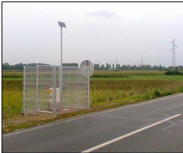
Figure 1. Automatic traffic counter based on inductive loops
