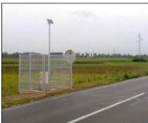
Figure 1. Automatic traffic counter based on inductive loops
